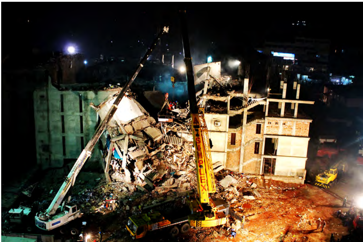
The remains of the Rana Plaza building collapse in Bangladesh.
