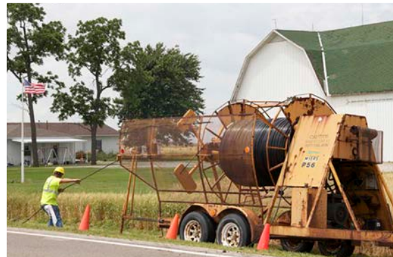
Workers for Com Net, Inc. and its wholly owned subsidiary Independents Fiber Network, installed nearly 700 new miles of broadband fiber to rural and underserved communities throughout western Ohio, thanks to federal stimulus funding under the American Recovery and Reinvestment Act. Their application for funding was part of a coordinated effort by Com Net, Inc., Horizon Telecom, OneCommunity and OARnet to create a comprehensive statewide plan to expand broadband infrastructure throughout the state.
